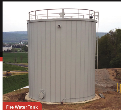
Fire Water Tank
