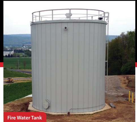
Fire Water Tank
